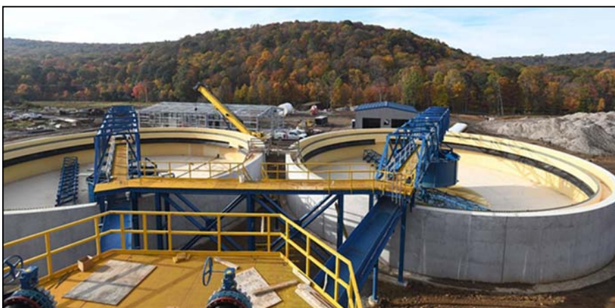
Blacklick Creek Treatment Plant: Project lead by PA BAMR for the treatment of 3 abandoned mine discharges: the Red Mill discharge, Vinton No. 6 "sister" boreholes, and the Wehrum Mine shaft discharge.
