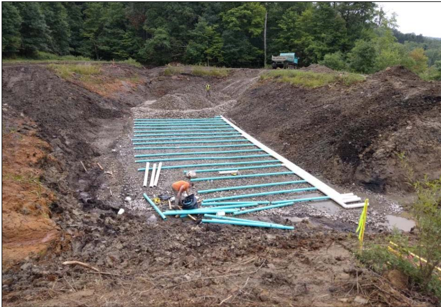
The Ferris passive treatment system, located in Venango Township, Butler County, in the Slippery Rock Creek Watershed, is shown at left when under construction. See article, front page, for information on its latest upgrade.
