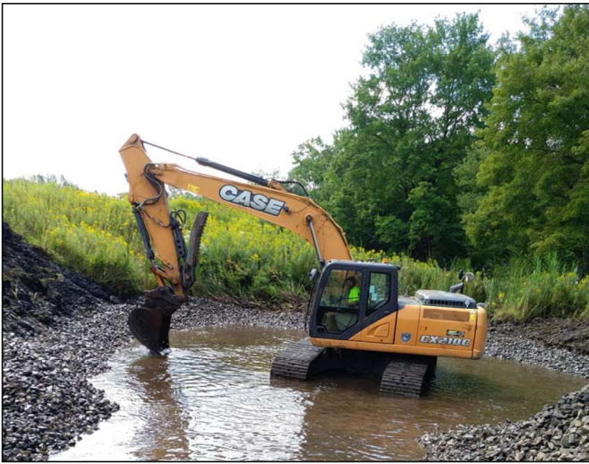
Cleaning the limestone at the De Sale Phase 1 Horizontal Flow Limestone Bed (HFLB). The De Sale Phase 1 passive system turns 20 years old this year, but keeps on treating water.
