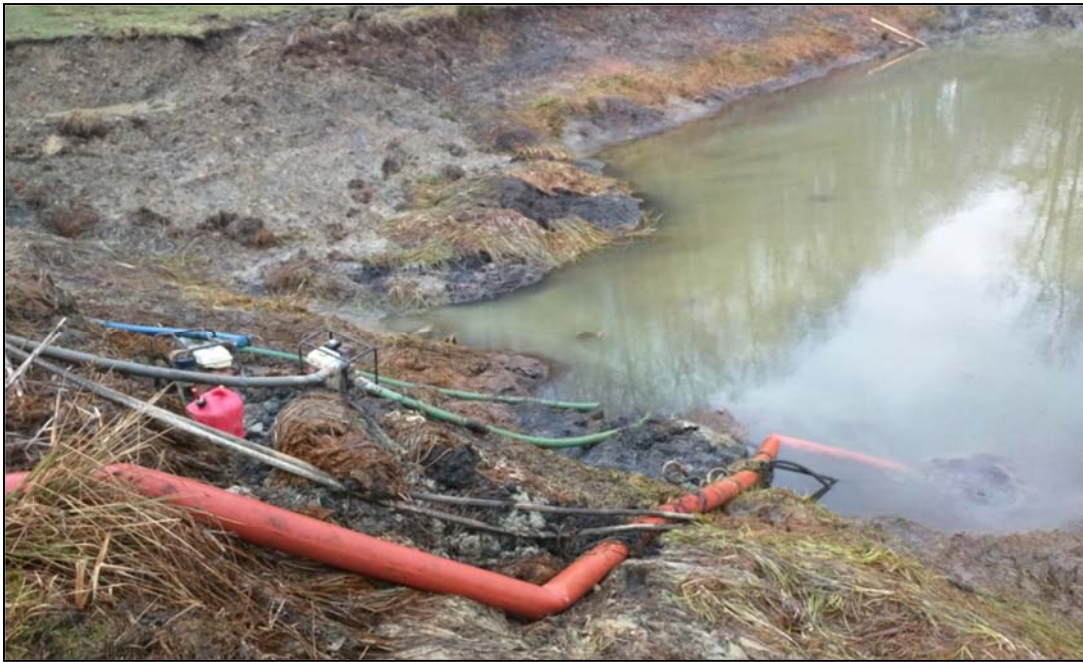
The vertical flow ponds at the Ferris Passive Treatment System Complex were pumped down to gain access to the treatment media.
