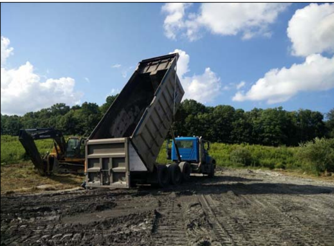
Placement of Mineral CSA (above) before replacing the vegetation and soil material. Maintenance began August 17.
