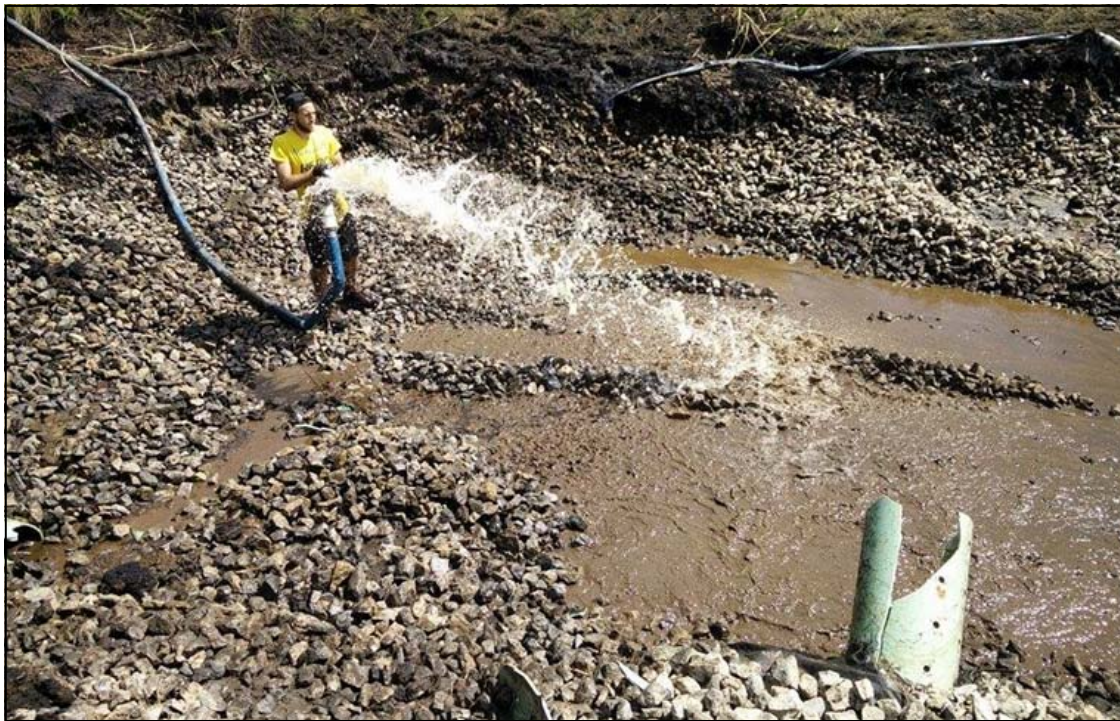
Brady Mahony cleans the stone at the Erico Bridge Passive Treatment System as part of the Slippery Rock Creek Watershed Renaissance grant awarded by the PA Department of Community and Economic Development. More about Brady next month...
