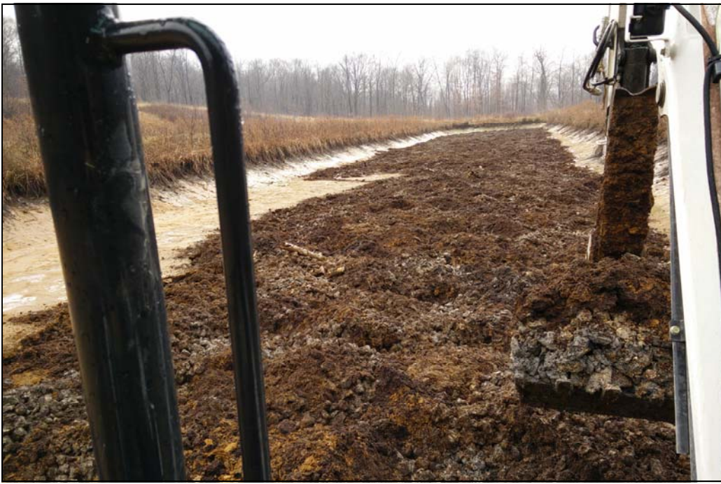
Ryan Mahony and Dan Guy from Bio-Most, Inc. recently completed some maintenance at the De Sale Phase I and Phase II treatment systems. This photo was taken by Ryan from the cab of the excavator as he stirred the treatment media at De Sale Phase II.
