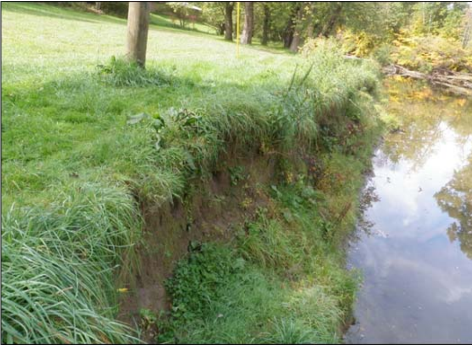
Active erosion of the streambank at the Slippery Rock Creek Campground. The utility pole (upper left) was moved in June 2011 and previously was over 20' away from the top of the bank. In March 2013 the pole was only 5' away from the bank. Thanks to a PA DEP Growing Greener grant, a 500-foot long segment of this streambank will be restored. (See article on the first page for more information.)
