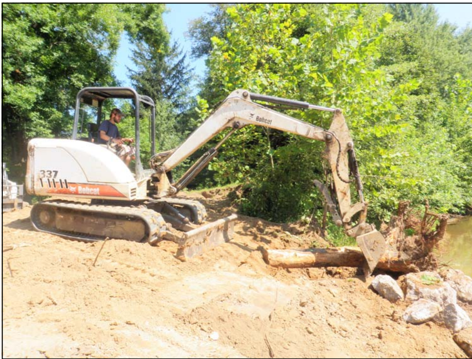
Ryan Mahony , of Bio-Most, Inc. and participant of the SRWC, uses an excavator to place a rootwad deflector along the bank of Slippery Rock Creek, Worth Township, Butler County, PA. More details to come in future issues of the Catalyst!
