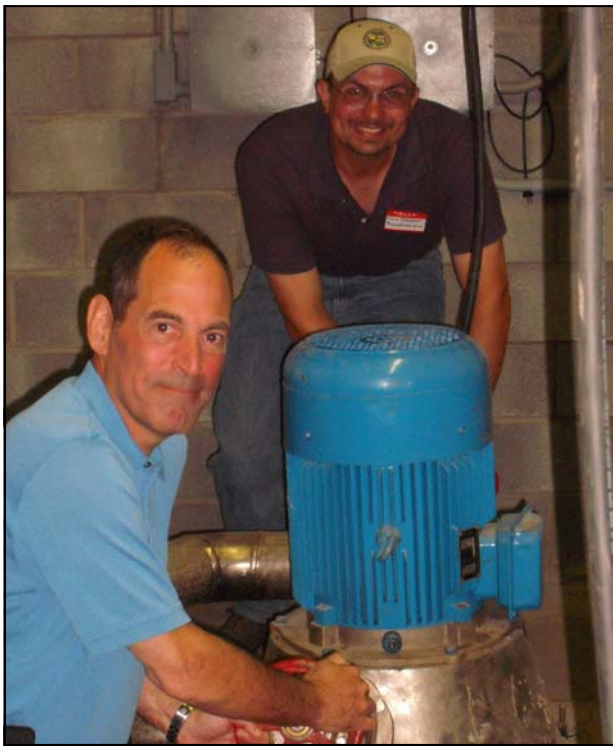
PA DEP Secretary Michael Krancer and Tim Danehy of BioMost, Inc. and SRWC participant, pose for a photo as the Secretary turns the valve to allow water to flow from the water treatment plant to the turbines to generate electricity at the Babb Creek Watershed Association's Antrim Micro-Hydropower Plant Dedication Ceremony held July 18, 2012. (Please see H.O.P.E. article on back page).
