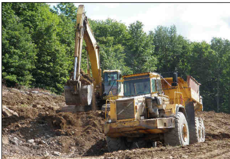
Wayne Fuchs, excavator operator for Quality Aggregates, Inc., loads a rock truck being driven by his daughter, Lindsey.
