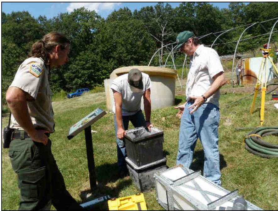
Dr. Phillip Sibrell, engineer, US Geological Survey, and Wil Taylor and Dale Margus from the Jennings Environmental Education Center, discuss installation and research efforts relating to a pulsed diversion well for AMD treatment. (Stay tuned!)
