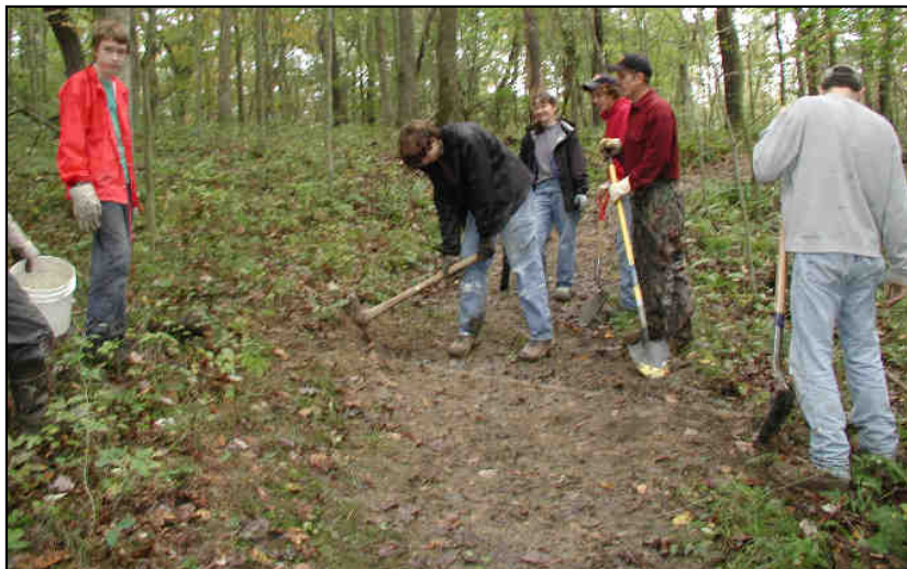
One crew built water bars to divert runoff and control erosion on steep trail areas
